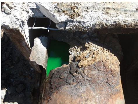
Fig. 1. Illustration of a pipe breakage accident.
